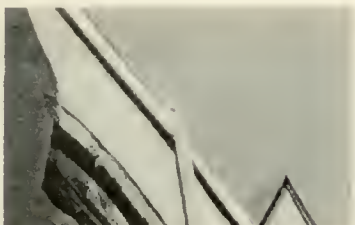
Figure 9 Disconnection of leader at east end of main sanctuary
